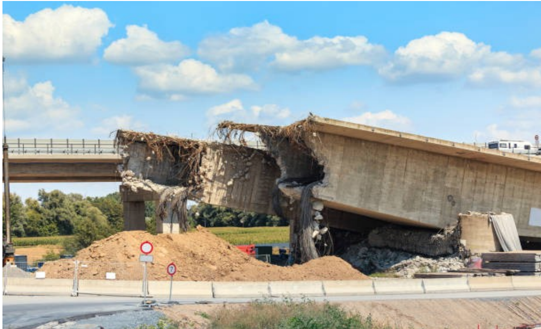
Image Credit 03: istockphoto frantic00 (Destroyed road bridge)
