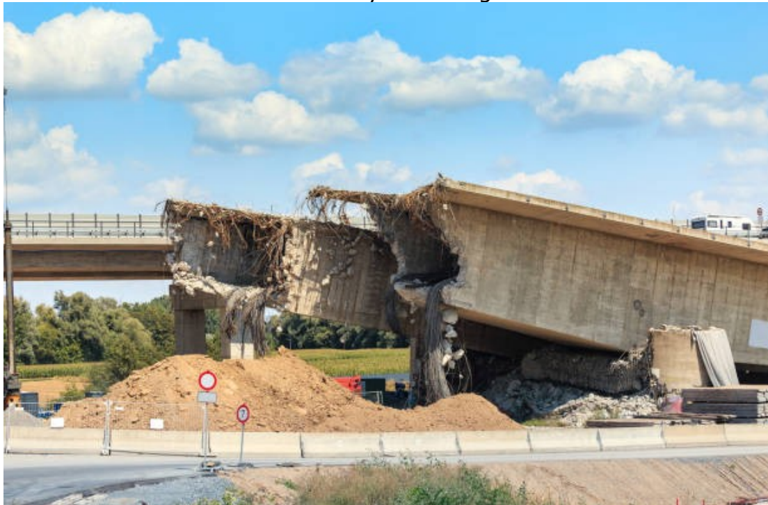
Image Credit 03: istockphoto frantic00 (Destroyed road bridge)
