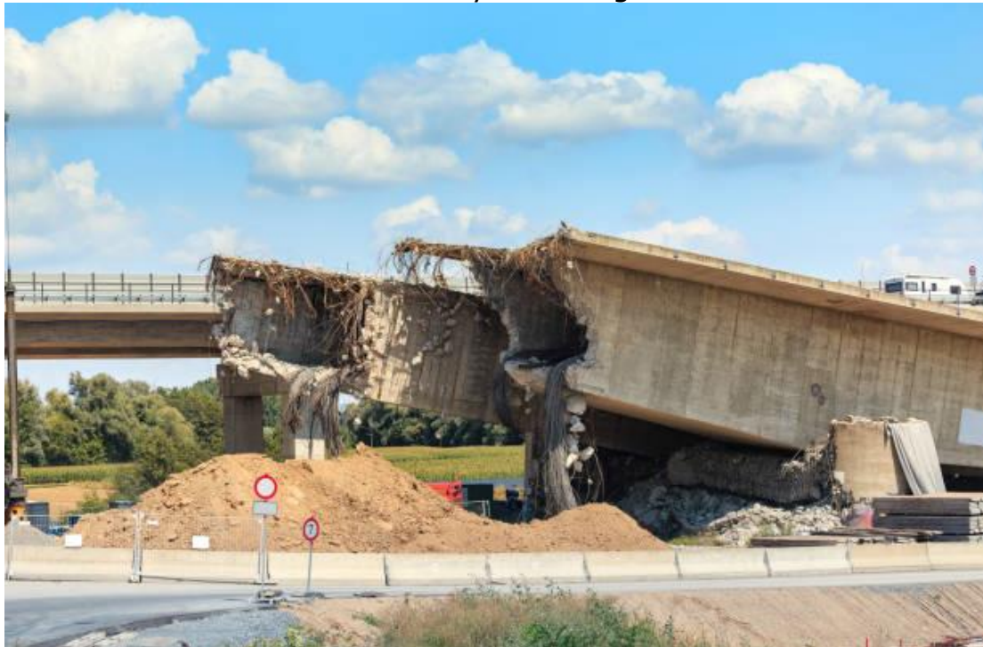
Image Credit 03: istockphoto frantic00 (Destroyed road bridge)
