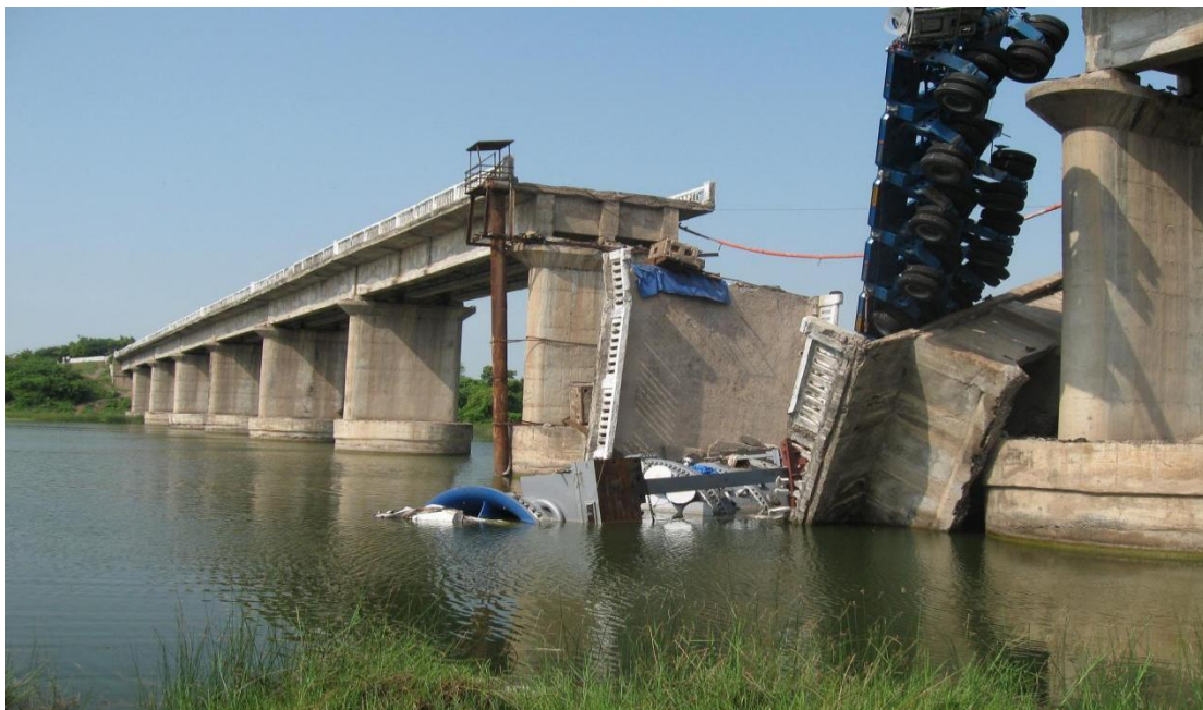
Image Credit 01: pixabay.com/photos/bridge-collapse-damage-312873/ /(Talaja Bridge)
