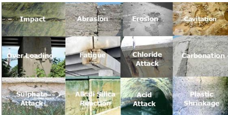
Figure 3: Various causes of bridge deterioration
