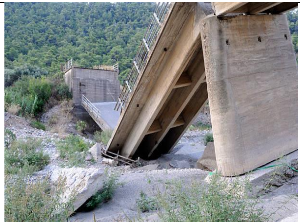
Bridge Collapse due to Earthquake
