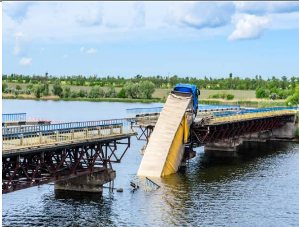
Bridge Collapse due to Flooding
