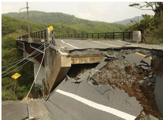
Bridge Collapse due to Landslide
